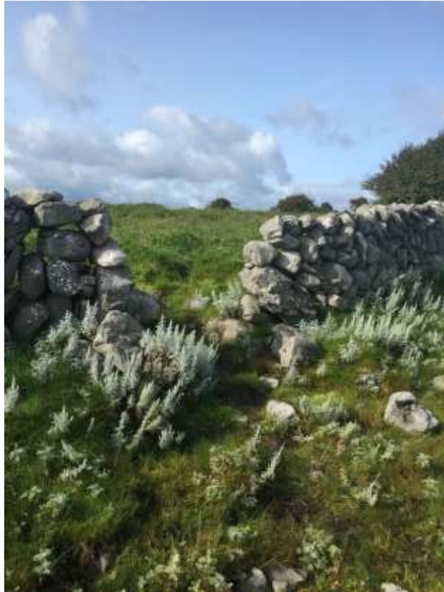
Photograph 1. Typical gap in limestone wall
