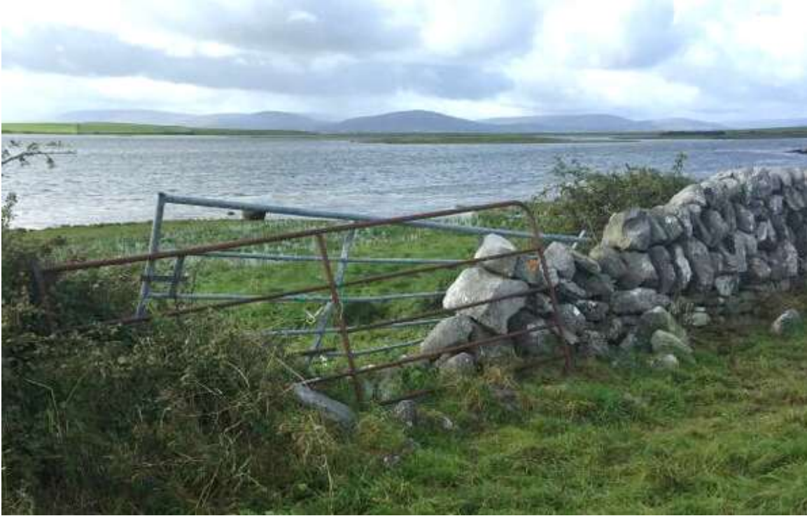
Photograph 2. Example of makeshift gate in wall which will be replaced by functional gate.
